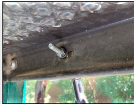
Priority 3 – protruding bolt
