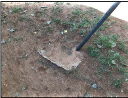
Priority 1 – exposed concrete footer
